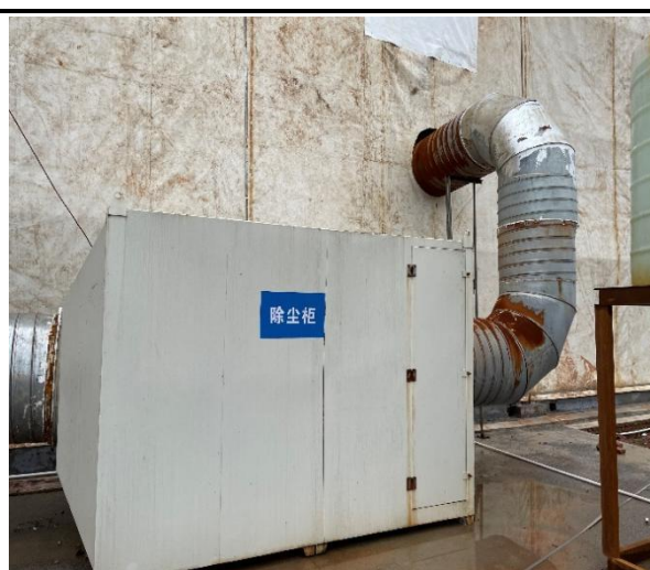
负压大棚尾气处理除尘柜
