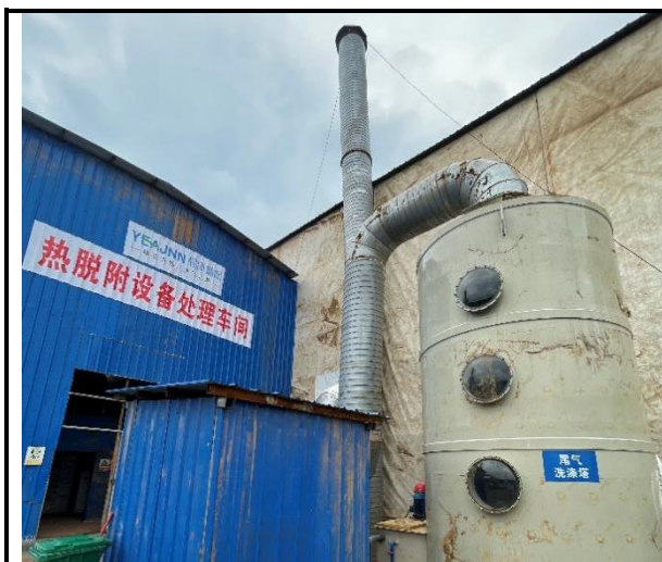
负压大棚尾气喷淋塔+15m 排气筒
